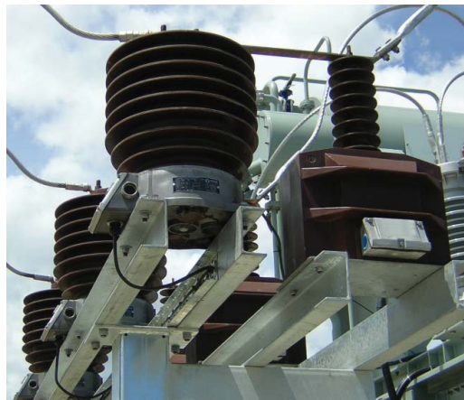
> 36 kV Current transformers (CR) and voltage transformers (UR). Revenue metering. Electronet Services (New Zealand).
