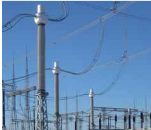
1. 765 kV Current transformer. RAO-FSK (Russia).
