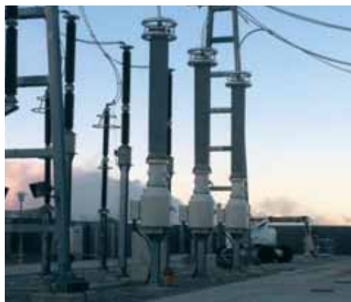
4. 420 kV Inductive voltage transformer. R.E.E. (Spain).
