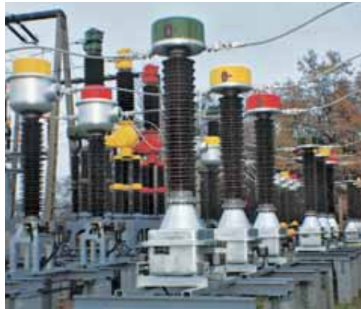
1. 123 kV Inductive voltage transformers (Bosnia).
