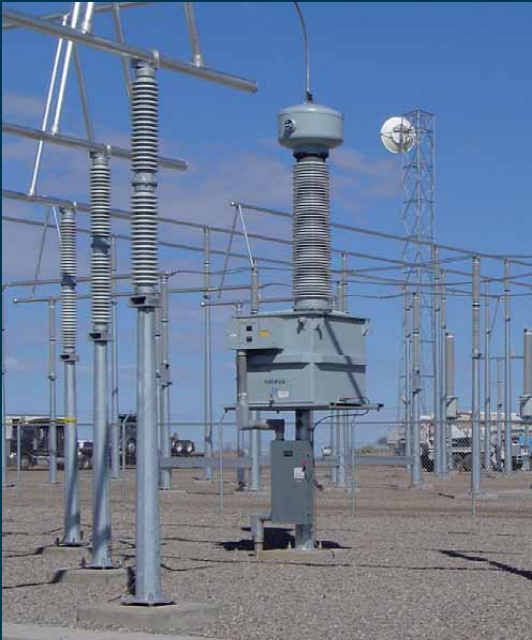
› 245 kV Transformer for substation auxiliary services, model UTP. Coyote Switch (USA).
