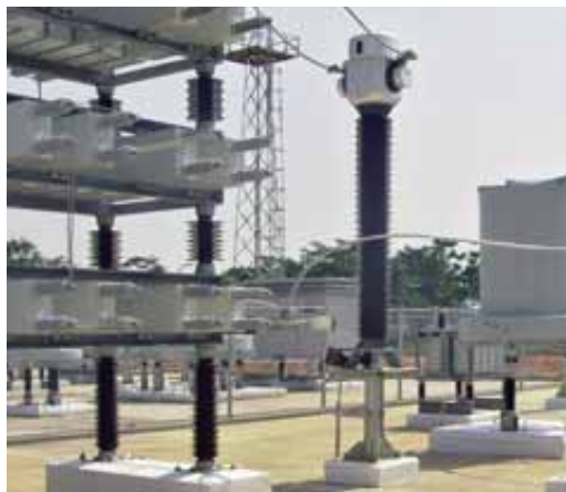
2. 245 kV Current transformer protecting capacitor bank (India).
