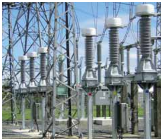
2. 123 kV Inductive voltage transformers. Transpower (New Zealand).
